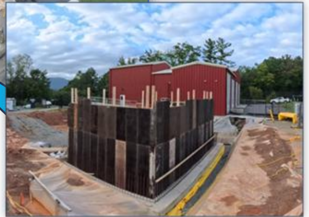
New clearwell to replace two smaller clearwell boxes.
